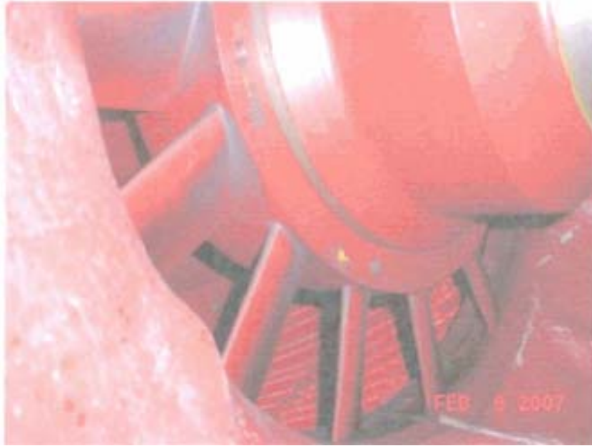
View of the generator rotor and stator and the exciter end.
