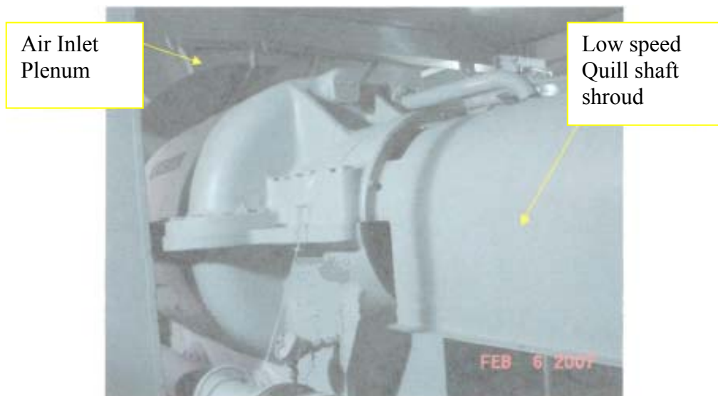
View of the low speed quill shaft shroud, coupling at the gearbox end and the inlet plenum.
