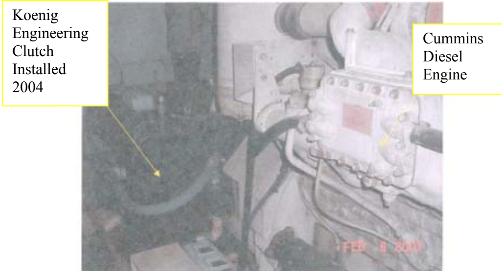
Diesel Start Pack as viewed on the north side looking towards the exciter.
