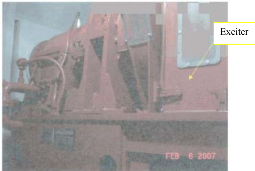
Exciter as viewed on the north side looking towards the generator.
