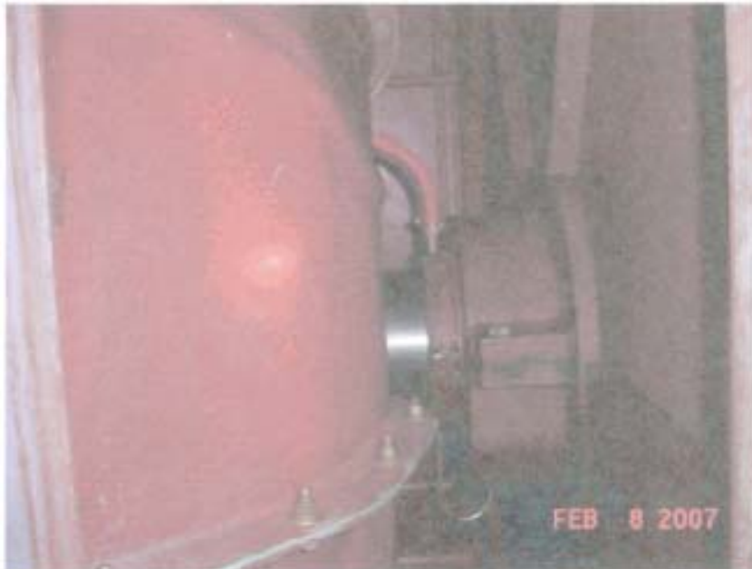
View of the generator bearing at the exciter end.
