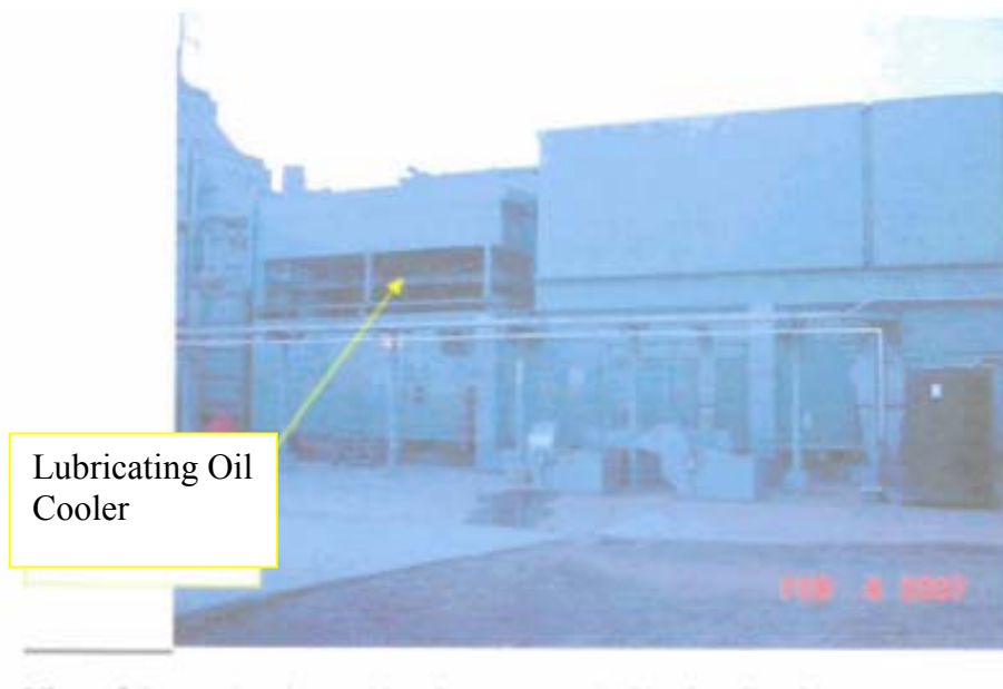
View of the combustion turbine from the north side showing the lubricating oil cooler.
