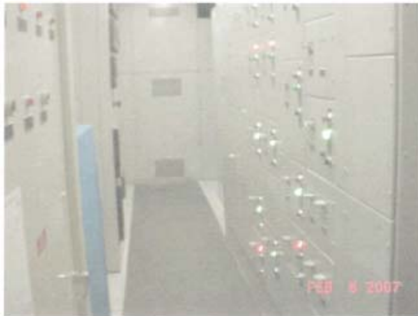
View of the MCC's located on the north side of the turbine and generator set.
